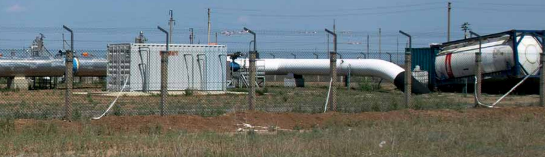
Caspian Pipeline Consortium pumping station in Atyrau. Photo: Rudolf ten Hoedt
